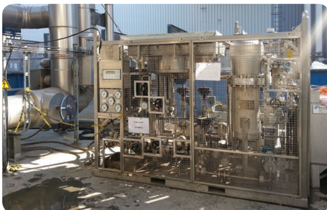
TFS state-of-the-art ATEX certified fluid conditioning rig.
